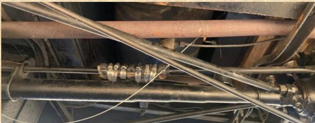
Above: A temporary fix on the Ruxtell rod using a wrench and some hose clamps
